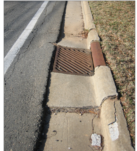
Above: An example of the uneven gutterpan/pavement seam on Concord Road, which essentially makes the functional portion of the bicycle lane less than two feet wide in some sections.
